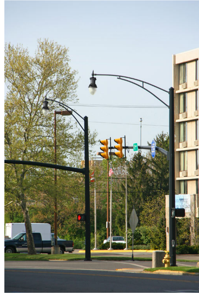
Traffic signal poles
