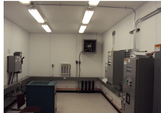
Interior of New Electrical Vault
