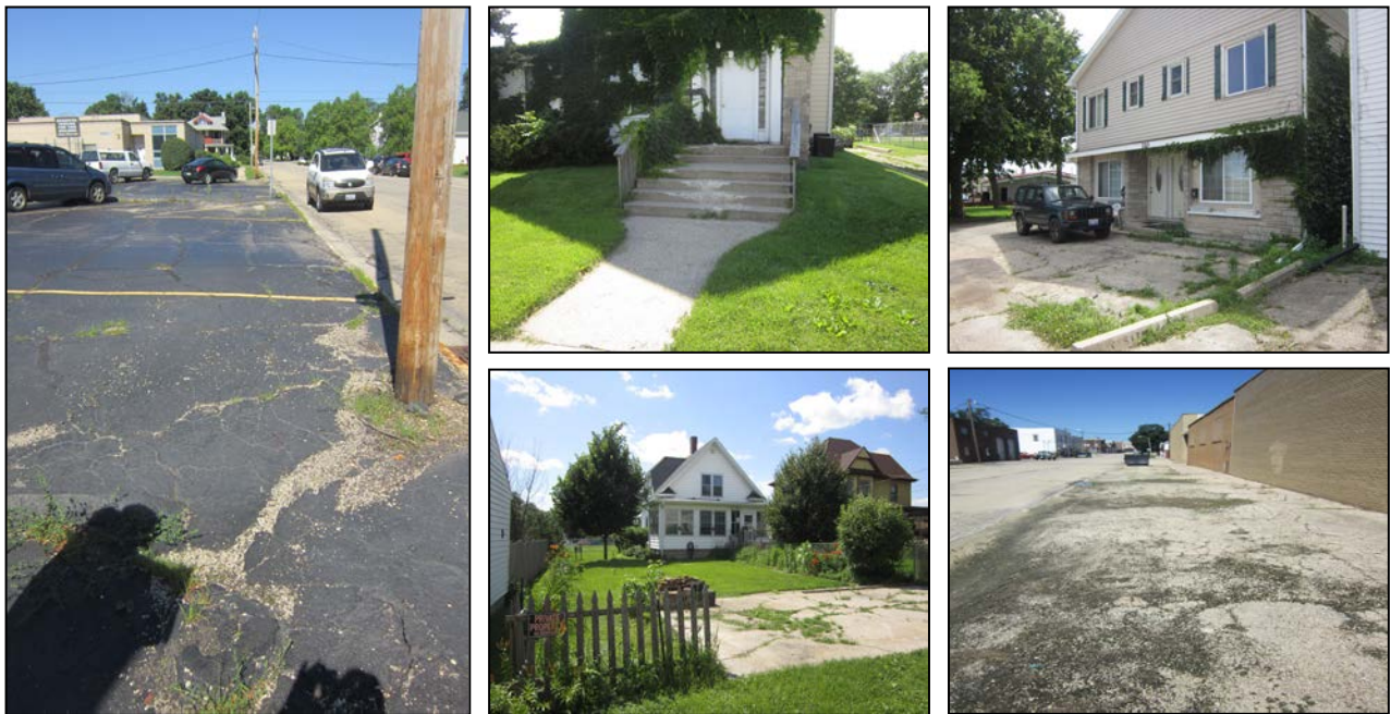
Examples of Site Deterioration
