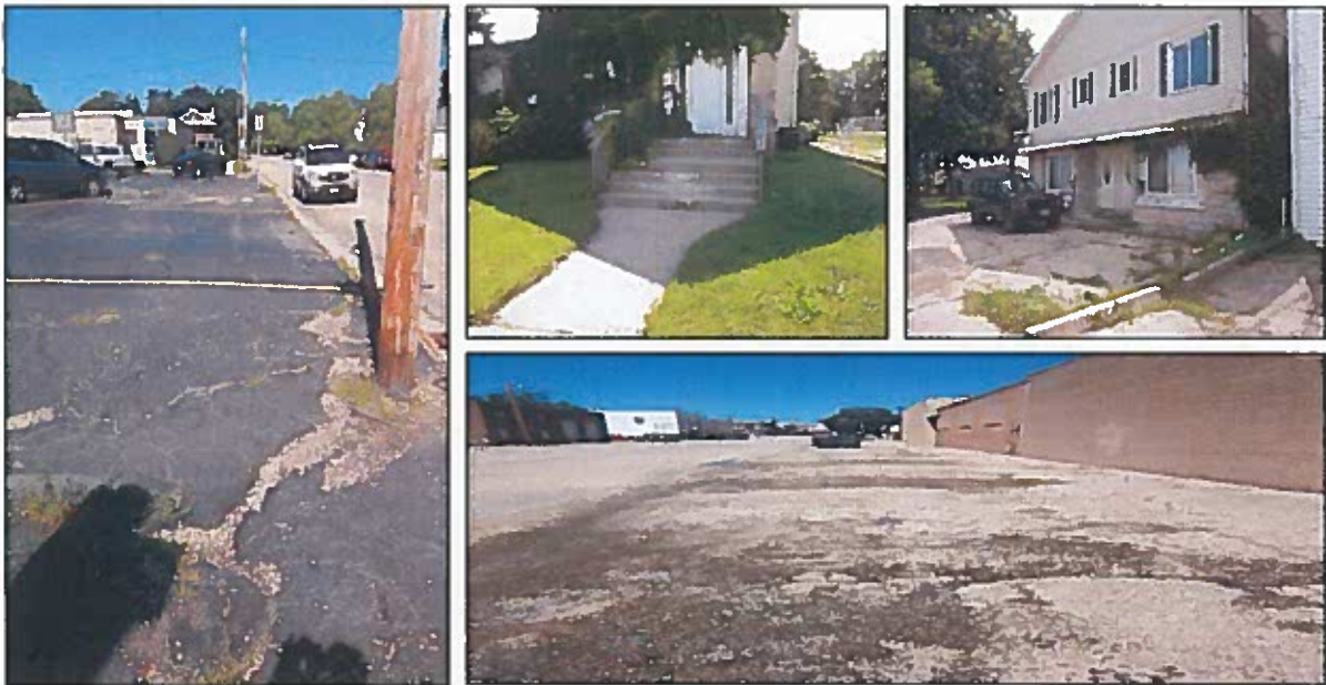
Examples of Site Deterioration
