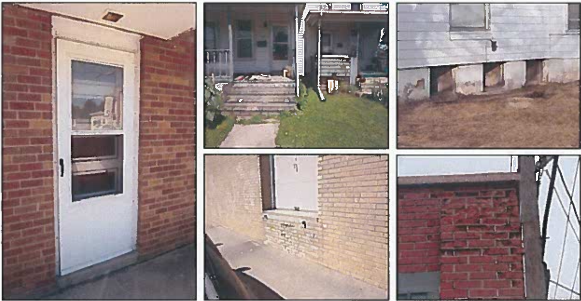
Examples of Building Deterioration
