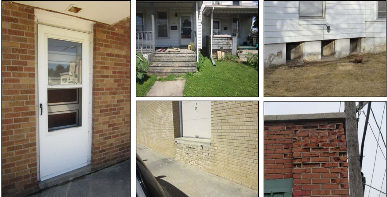
Examples of Building Deterioration
