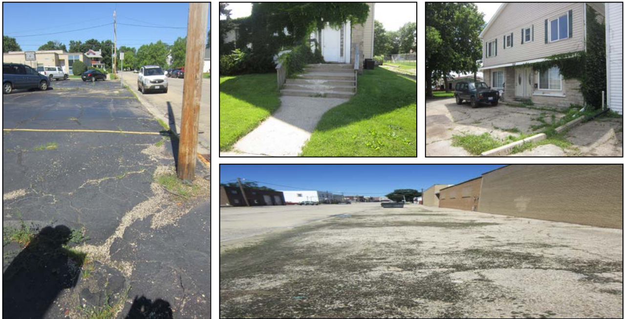
Examples of Site Deterioration
