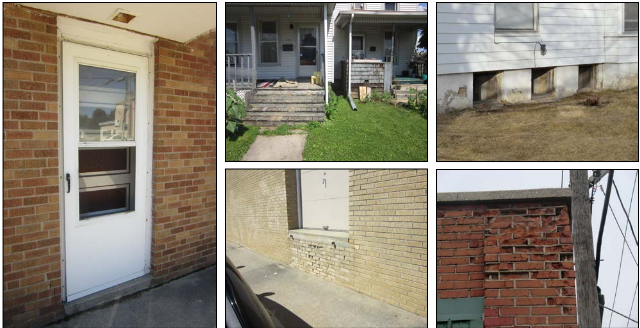
Examples of Building Deterioration
