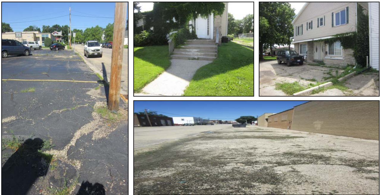
Examples of Site Deterioration
